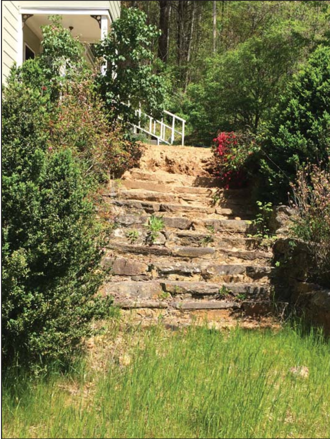
Photograph 1: View of original steps from the public right of way; looking east. (2016)
